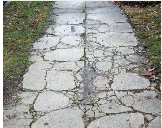
Poor = many cracks, unsmooth surface
